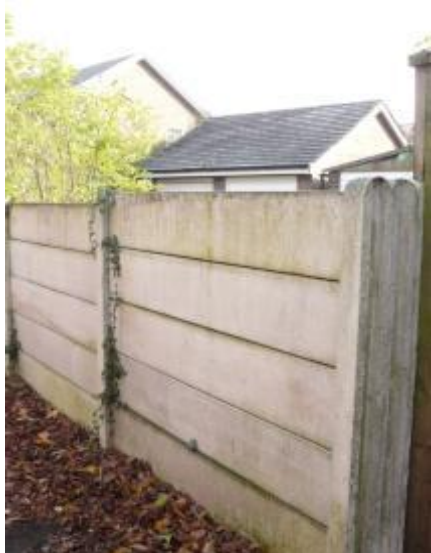
Photograph 44: Intrusive Concrete Fence on The Narrows
