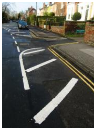
Photograph 47: Thick and high profile road marking
