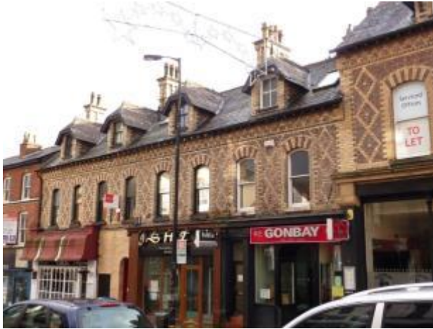
Photograph 40: Intrusive Permanent Awning
